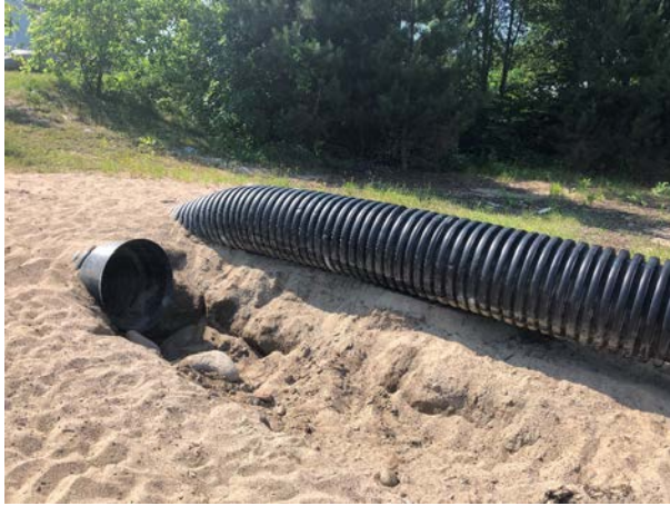
PHOTO 8 MATTAWAN STREET CULVERT AT HURDMAN STREET POST MAY 2019 FLOOD
