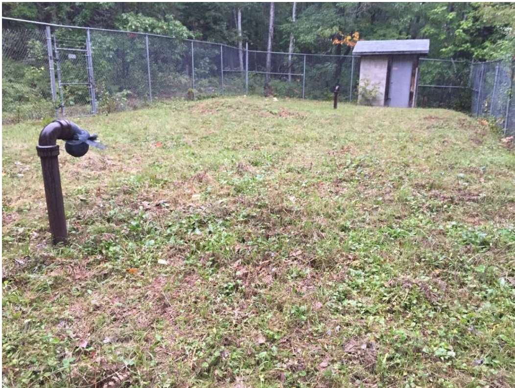
PHOTO 12 TOWN OF MATTAWA WATER RESERVOIR
