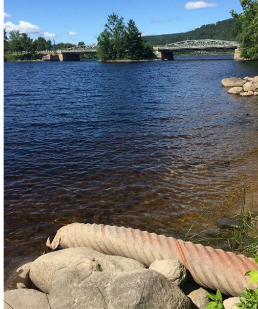
PHOTO 9 MATTAWAN STREET CULVERT AT PINE STREET POST MAY 2019 FLOOD
